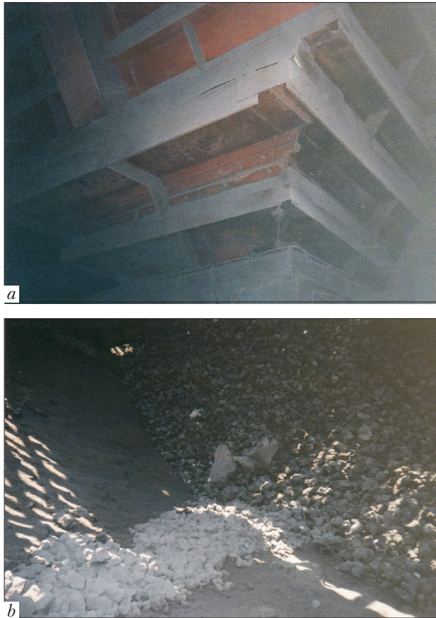
Fig. 2. Damage of steel hoppers for ore agglomerate storage: a – broken reinforcement ribs; b – destruction of brickwork
