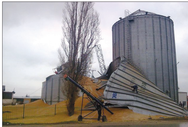
Fig. 1. Failure of steel grain storage facility
